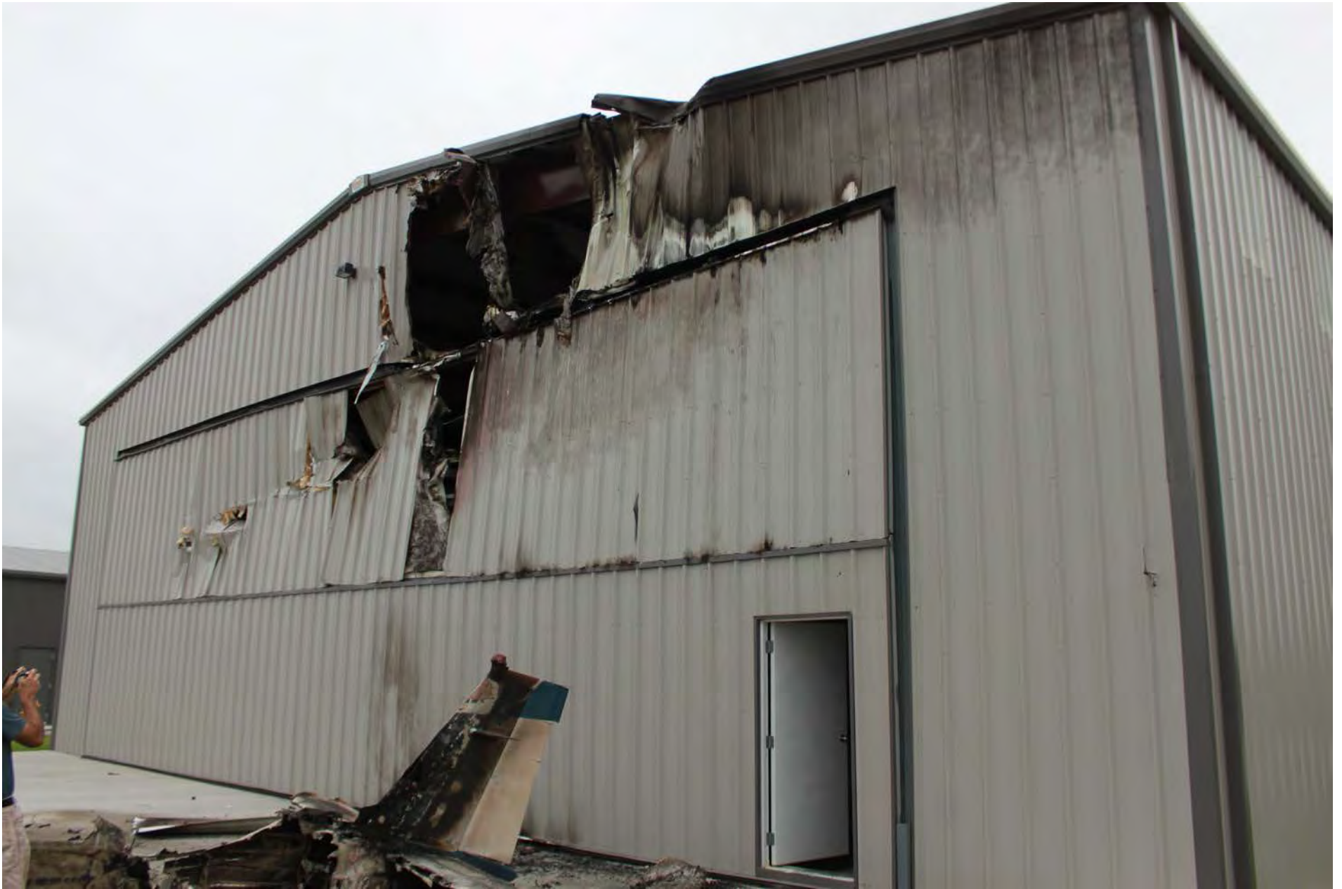
Photo 3 – View of hangar that was struck
