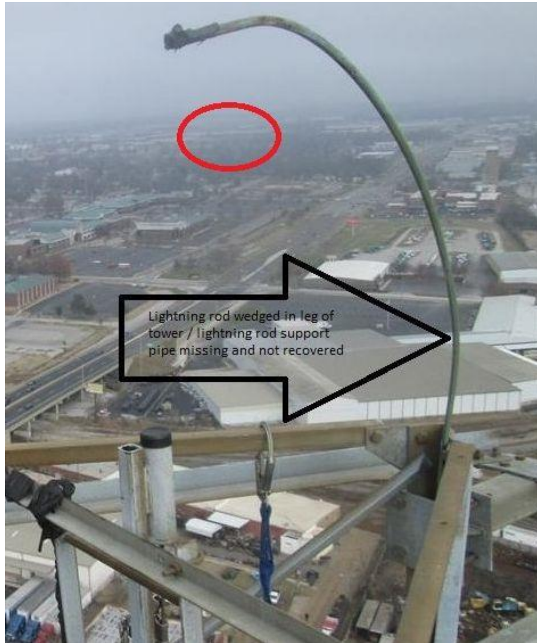
Photo 4 – View of separated lightning rod – photo dated December, 2014 (Verizon Photo)
