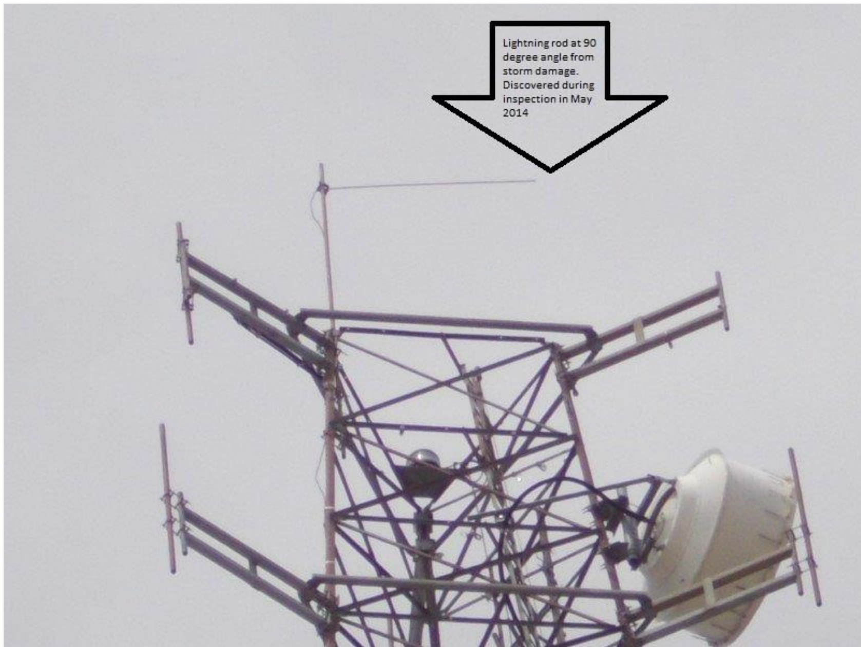
Photo 3 – Top of 367 foot tall cellular tower – photo dated May, 2014 (Verizon Photo)
