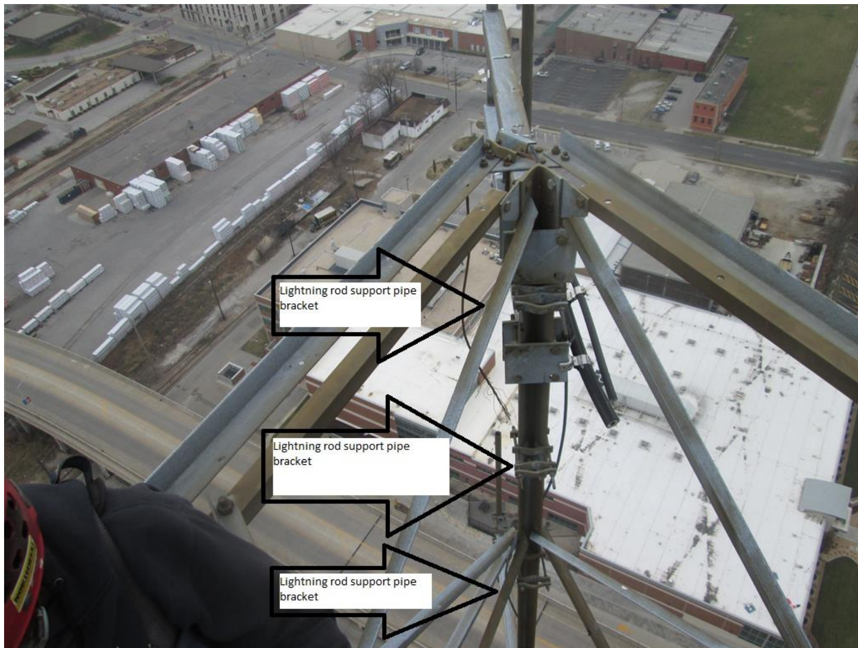
Photo 5 – View of lightning rod support pipe brackets – photo dated December, 2014 (Verizon Photo)
