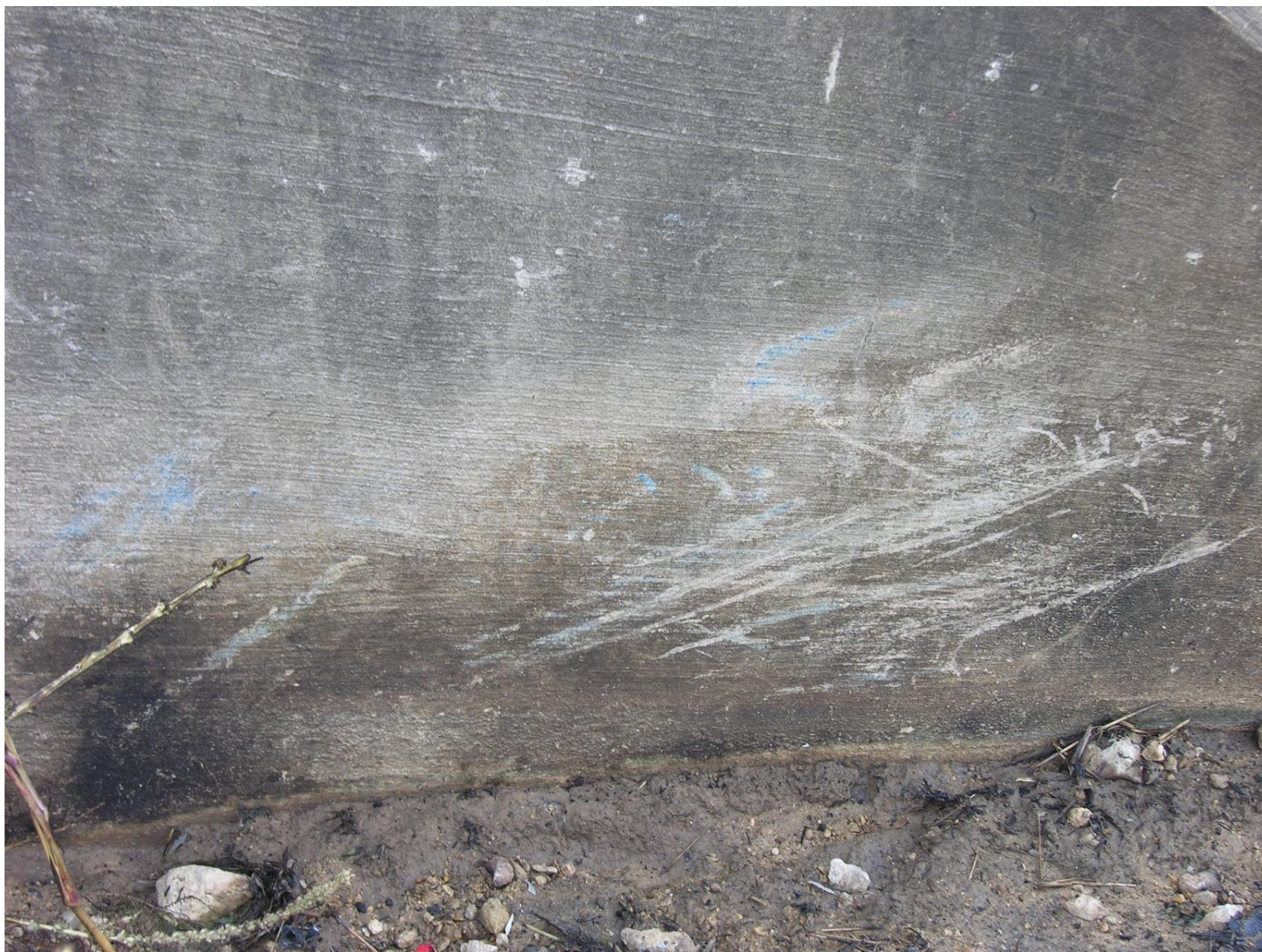
Photo 5 – Close-up view of the south sidewall of the concrete box culvert (NTSB Photo)
