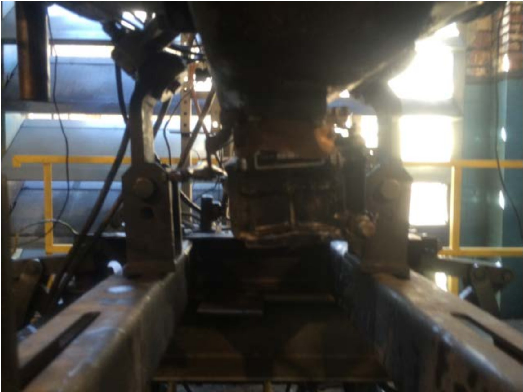
Photo 13 - View of the repaired carburetor mounted on the accident engine within the test cell.
