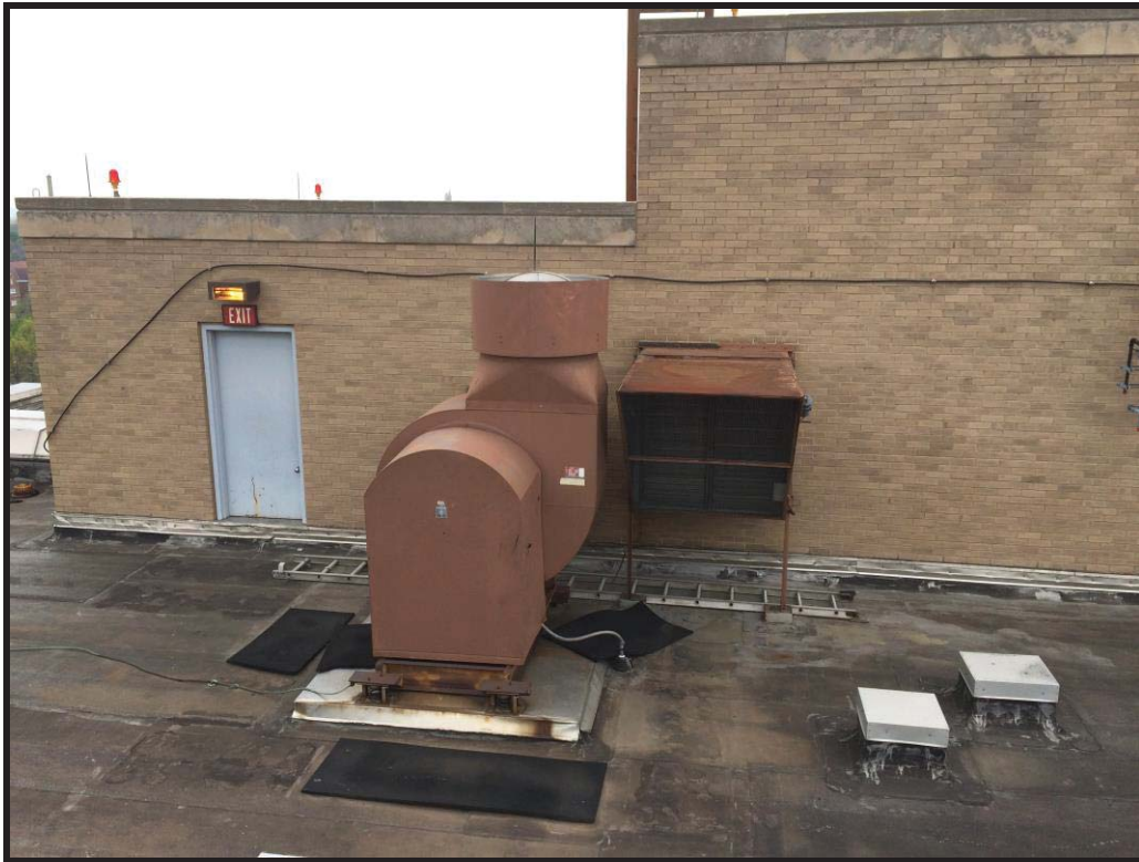
Figure 23: Building Ventilation Equipment (Table 2, Item 14)
