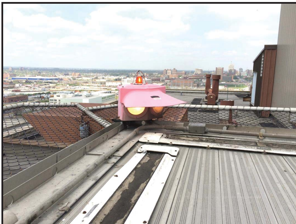
Figure 19: Raised TLOF Perimeter/Flood Light (Table 2, Item 13)
