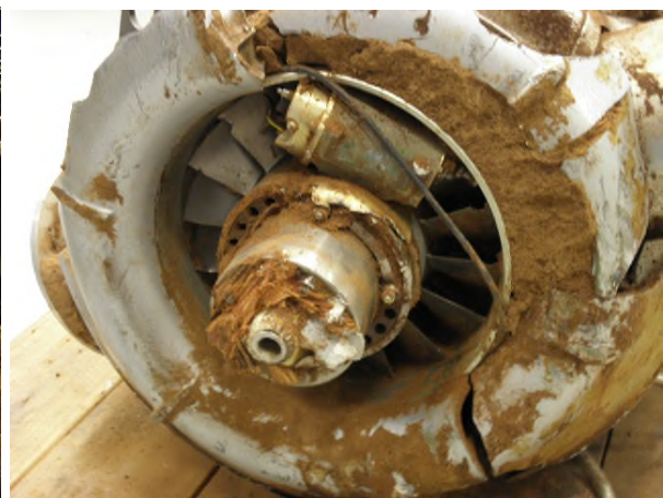
Photo No. 4, Compressor inlet
