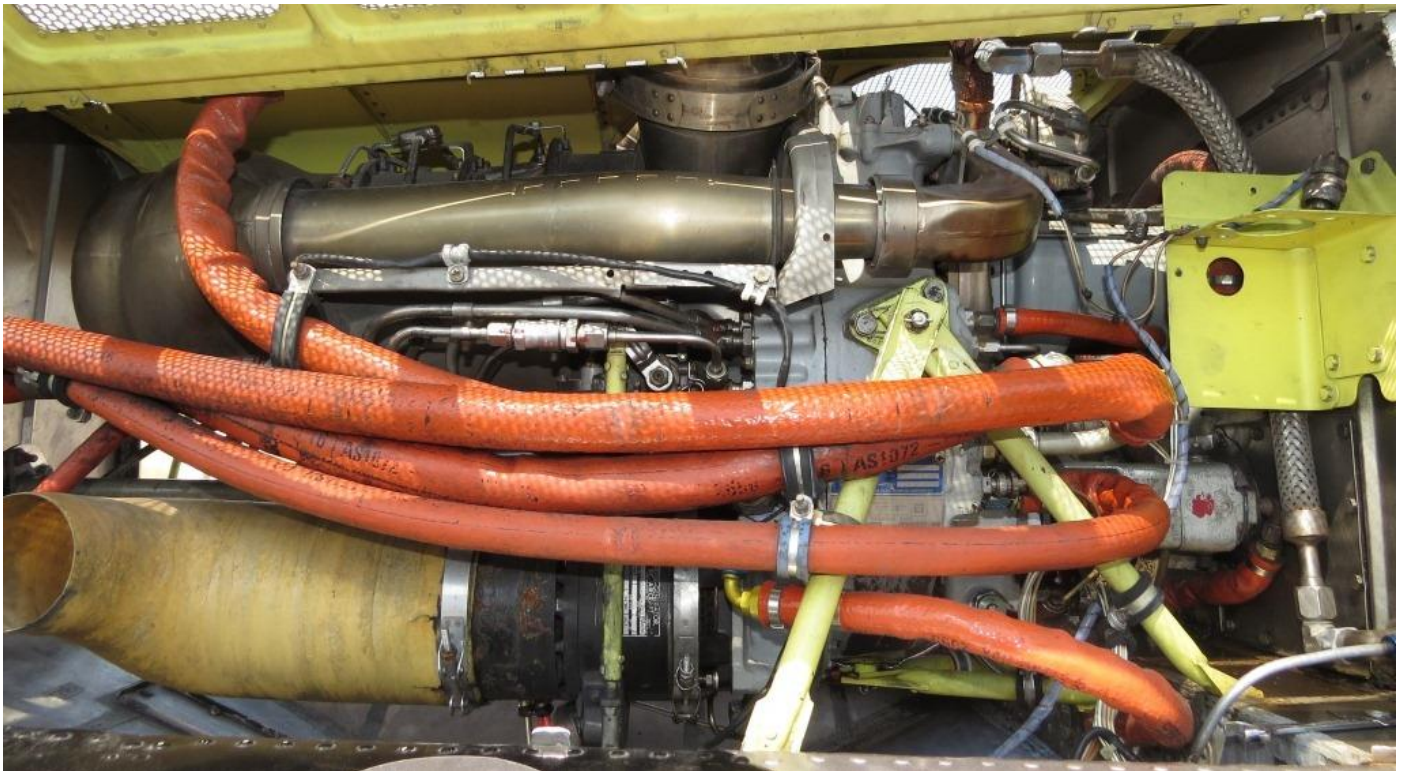
Engine as Installed – Right Hand Side
