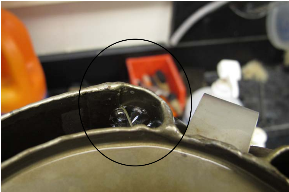
Figure 15. Photograph of leak in heat muff end weld. The leak (circled in black) is made visible by the bubbling leak detector liquid.
