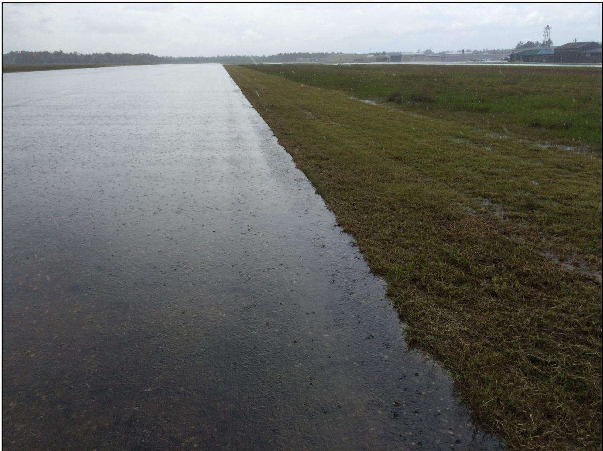
Figure 2b. Photo of west edge of KCXO runway 1 during a 0.5 in./hr. rain event.
