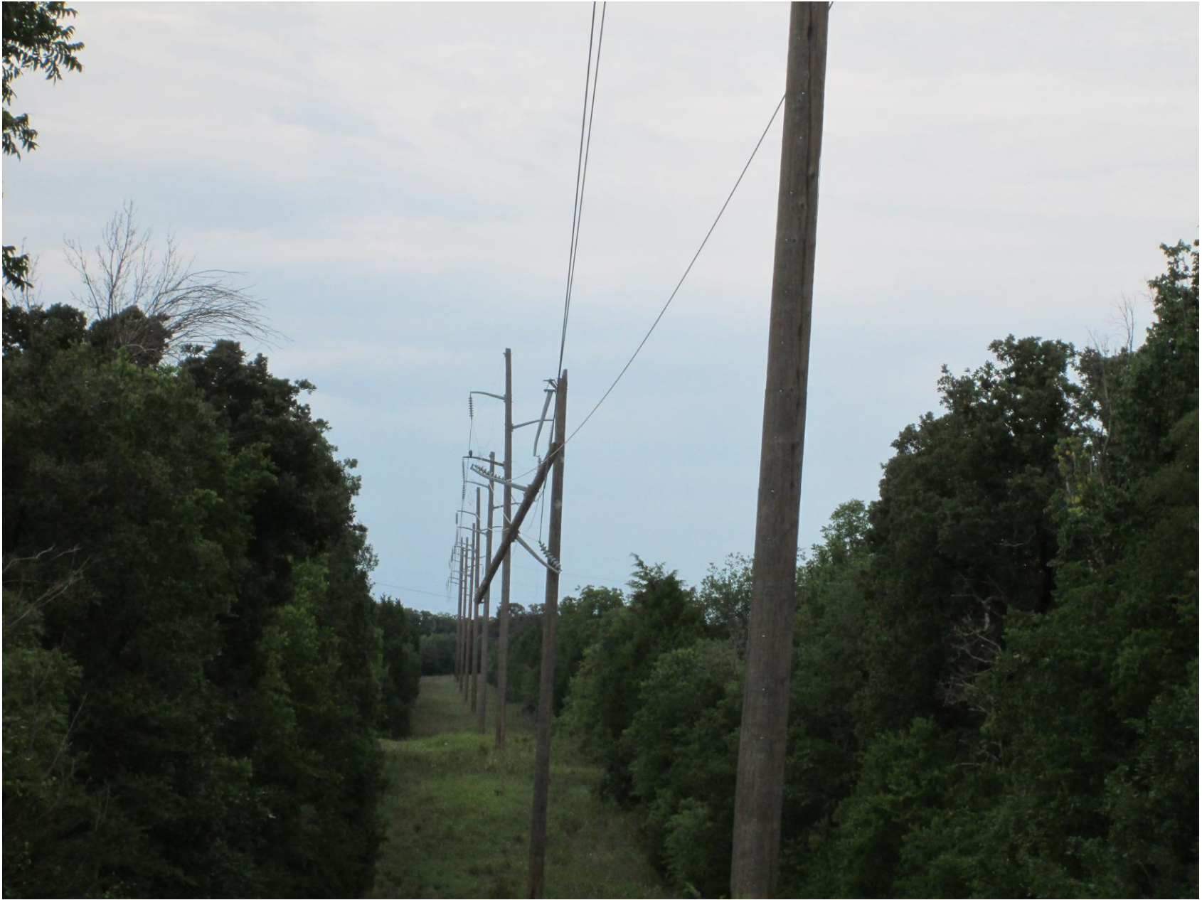
Photo 3 - A powerline is seen, with several cables strung along each pole. One of the poles is broken, near the top, and the cable appears to be pulled down.
