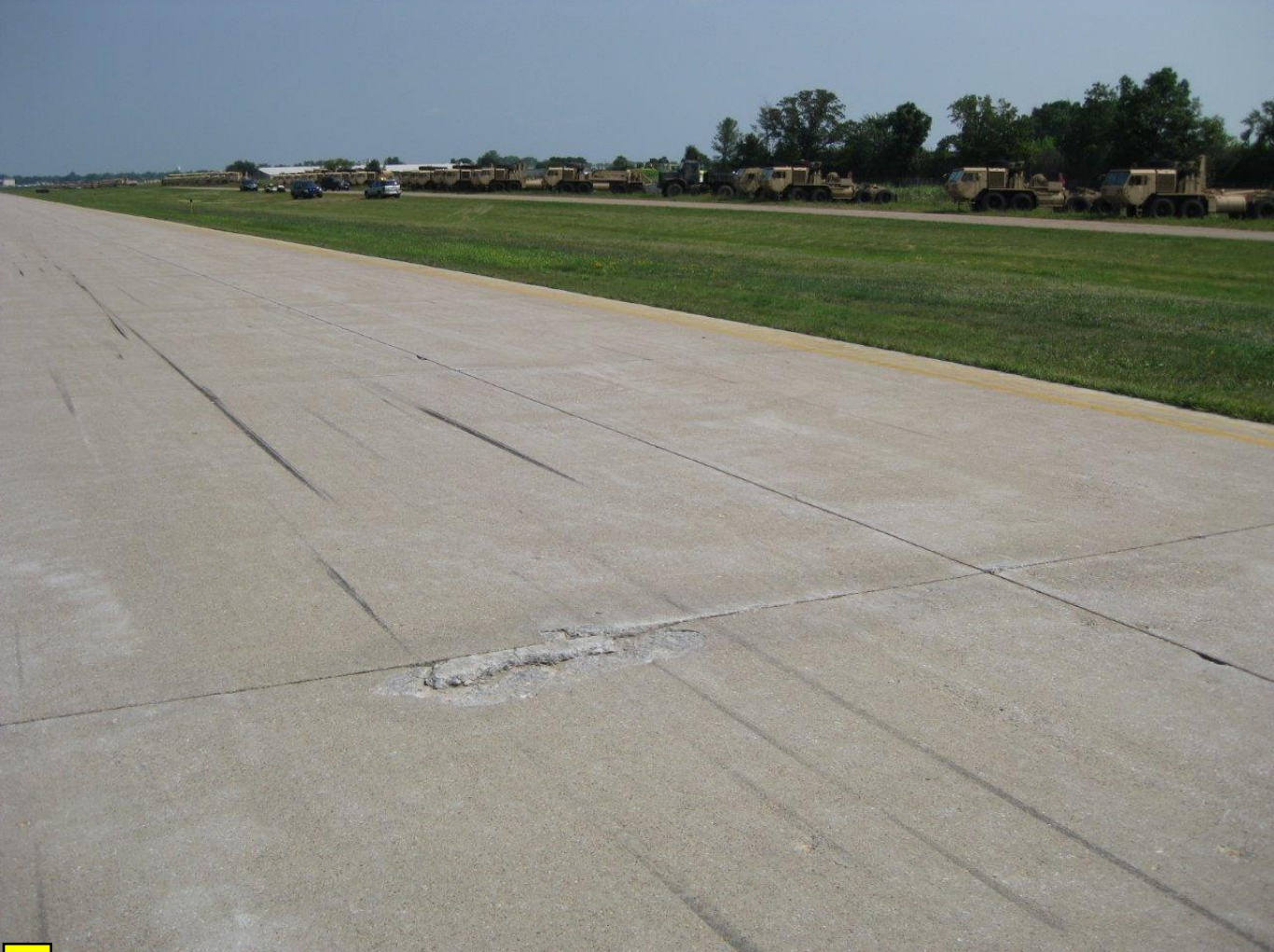
Photo 4 - Runway depression abeam path in grass
