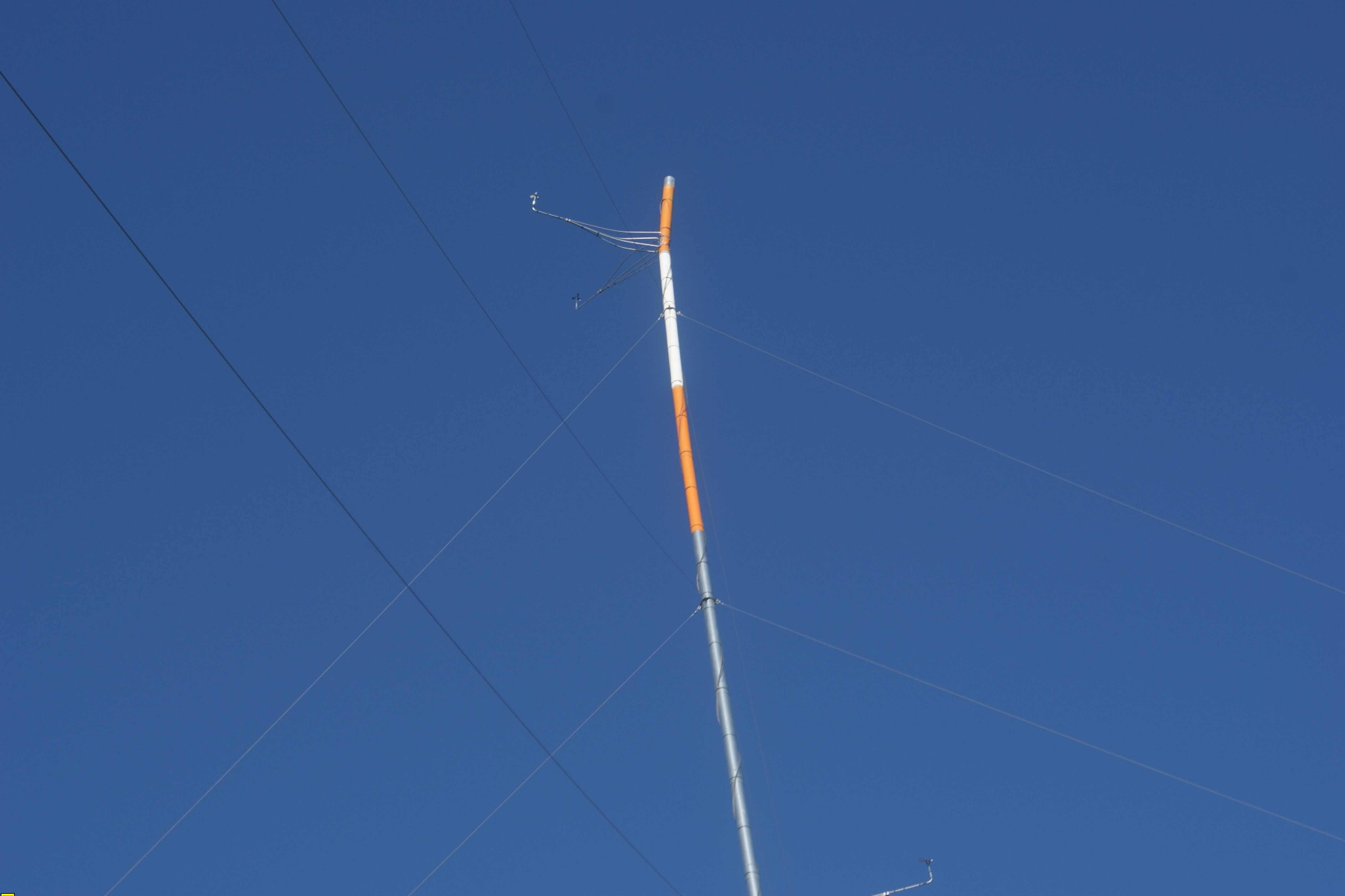
Photo 1 - Meteorological tower that was struck by N3159B. Note tower is bent and severed at the top.
