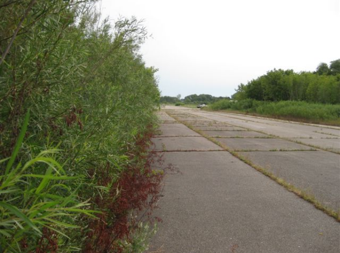
Photo 3 Closeup View of Overgrown Vegetation on the Side of the Runway
