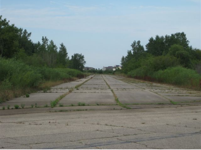
Photo 2 View of Runway with Overgrown Vegetation
