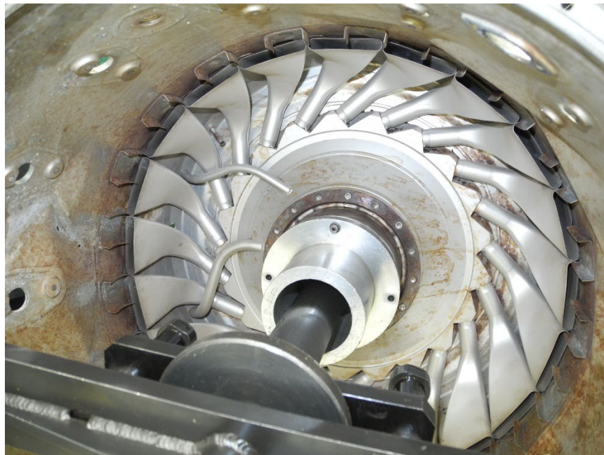
Photo 32 - GG Case Diffusers - Intact
