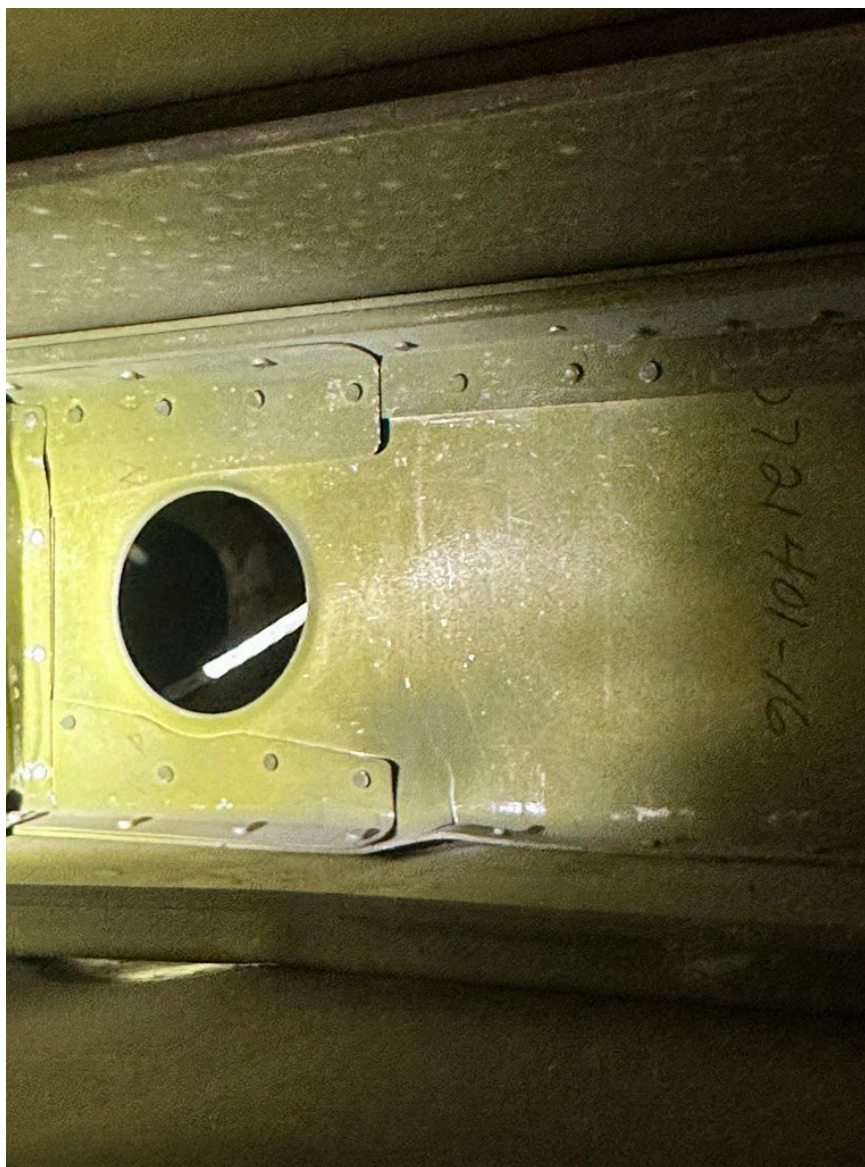
Photograph 3 - View of damage to right spar (Courtesy of pilot)
