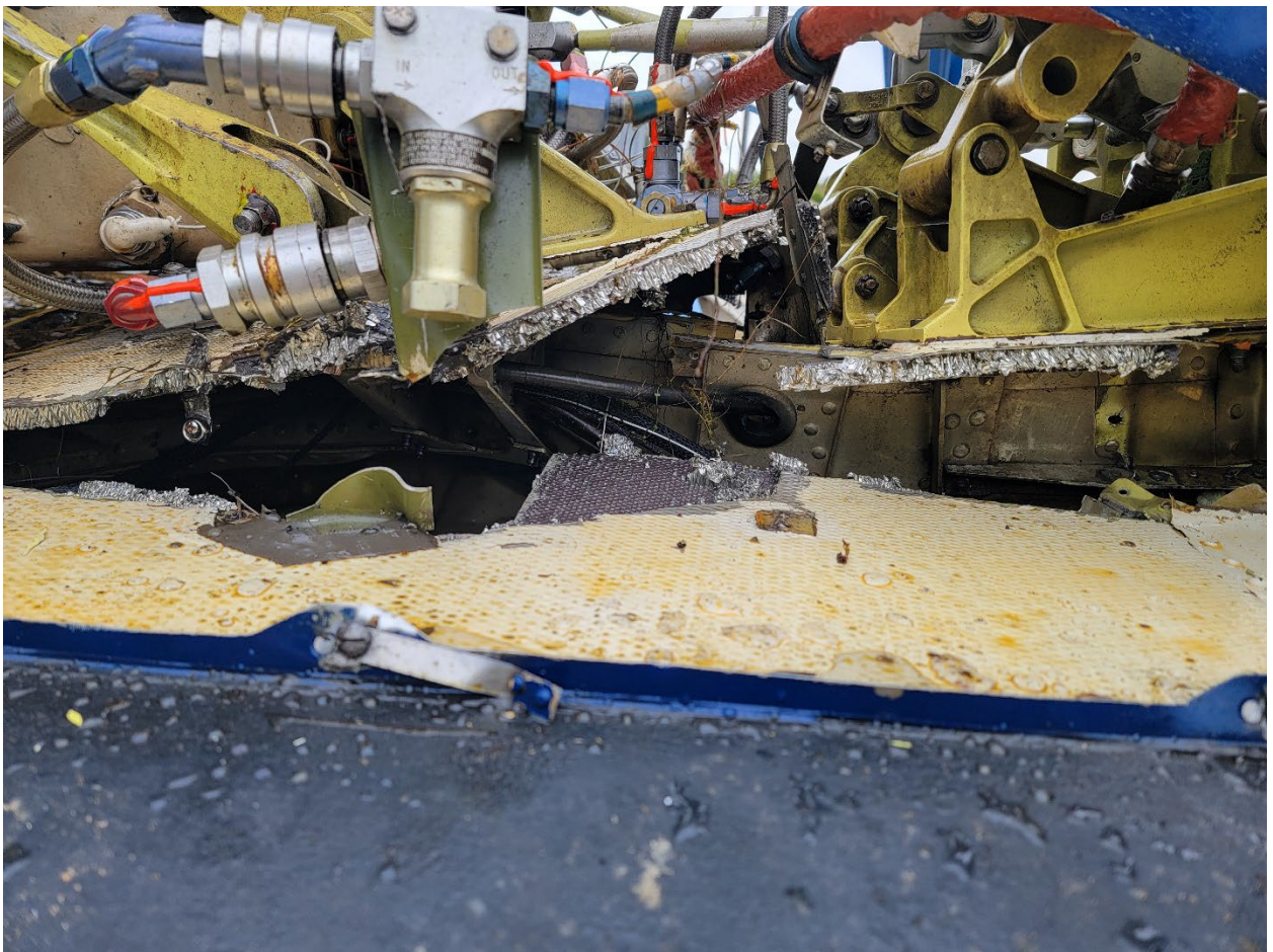
Figure 15 View of the right side damage to the floor below the main transmission and flight control servos.
