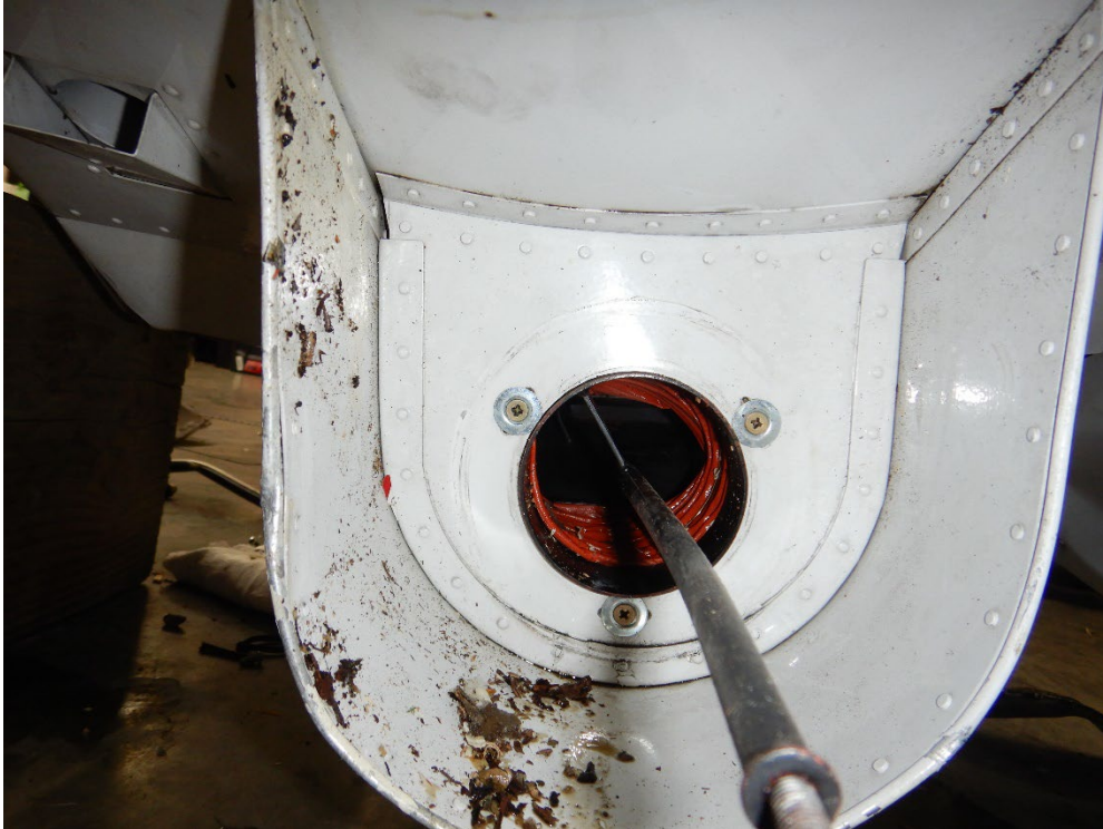
Figure 9 View looking into air intake with filter removed
