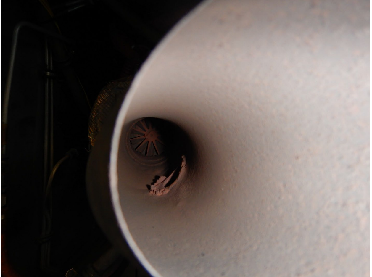
Figure 6 View into the exhaust to the turbo fan.
