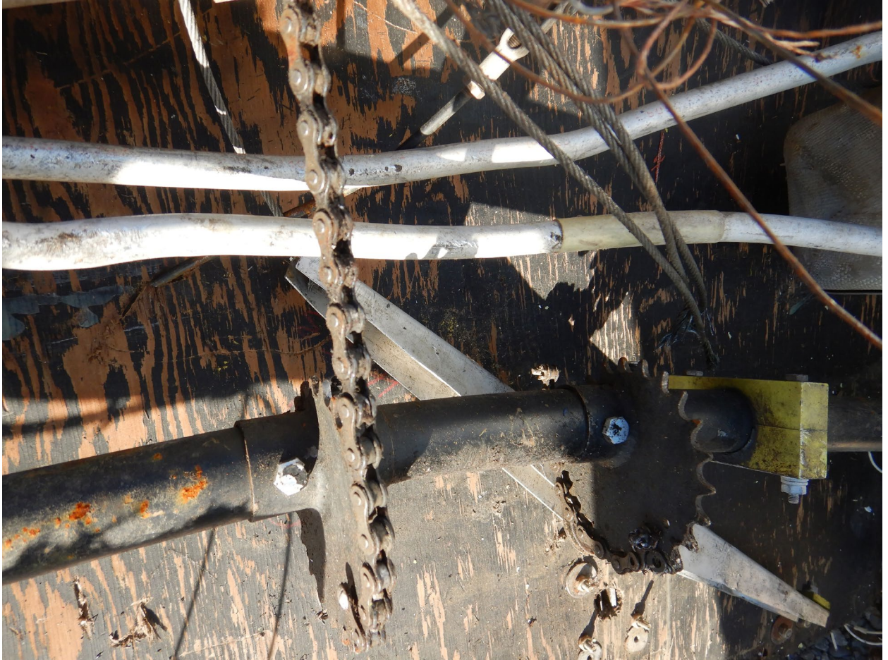
Figure 32. View of control cable breaks under the floorboard near the instrument panel area.
