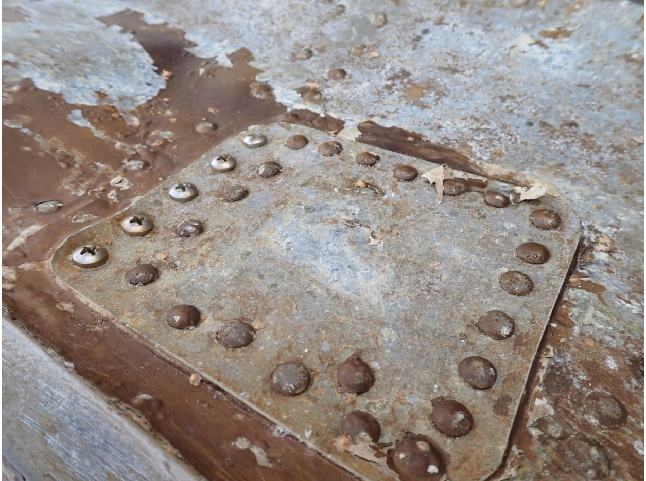
Figure 3 View of patch and screws on the hull of the right float (Photo courtesy of Textron)
