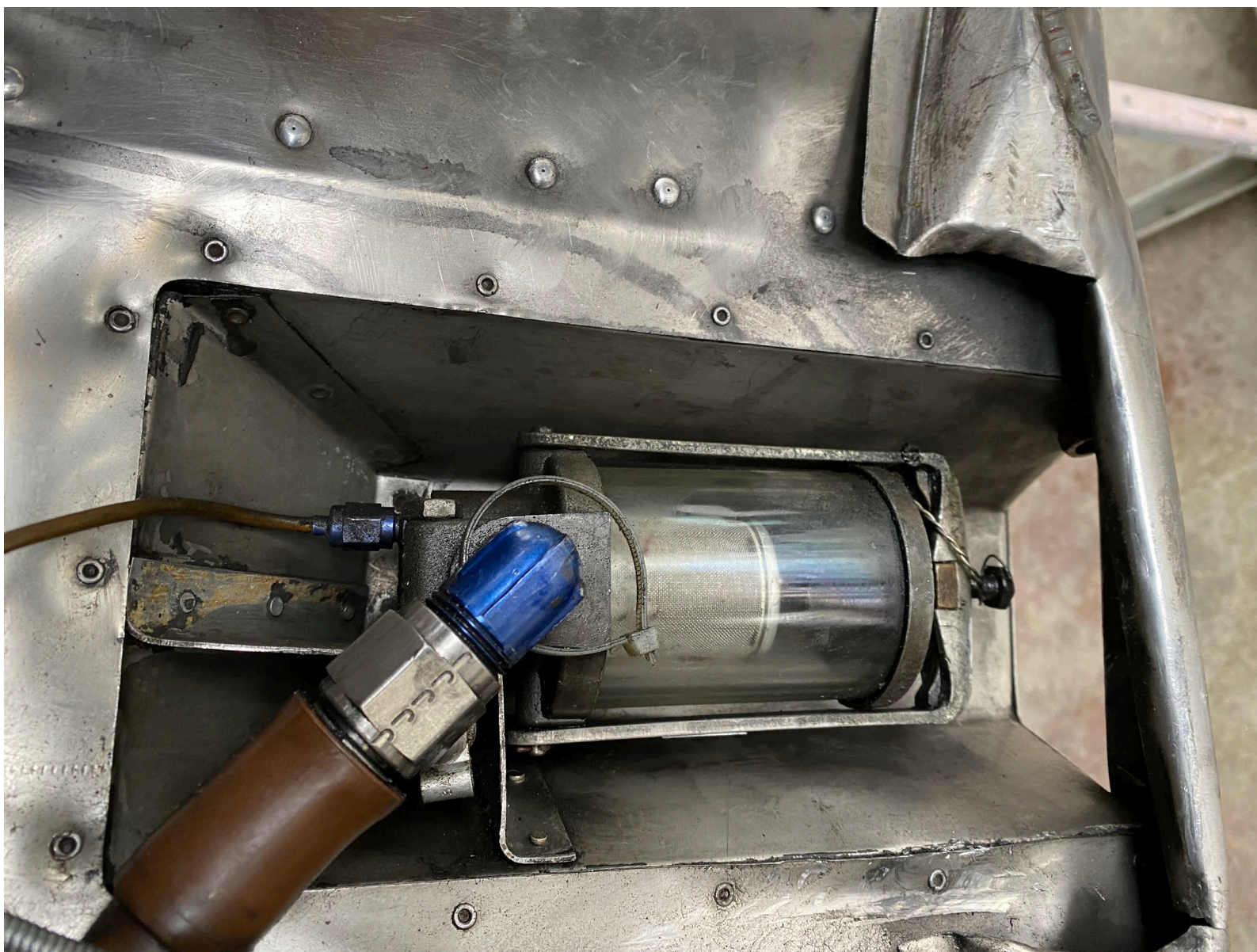
Photograph 6 - Fuel strainer (Courtesy of FAA)
