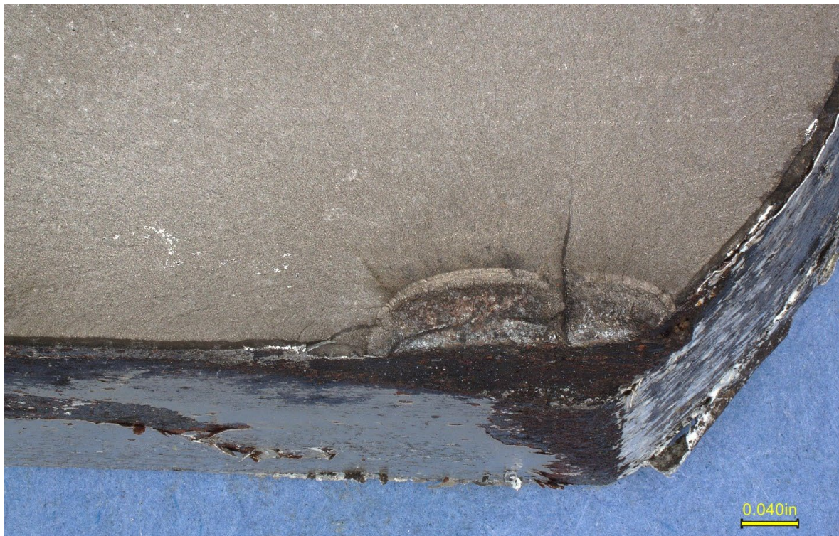
Figure 8. Closer view of the thumbnail cracks, after cleaning the fracture surface.
