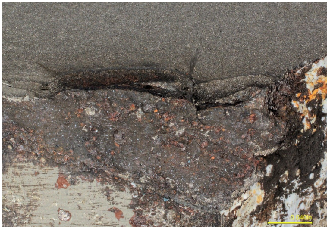
Figure 18. Corner of the crack initiation site, showing the corroded underside.
