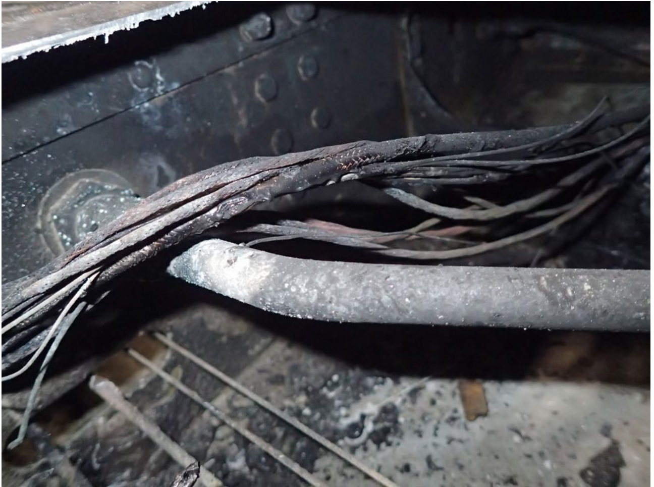
Figure 8 View of wire bundle crossing over fuel line.
