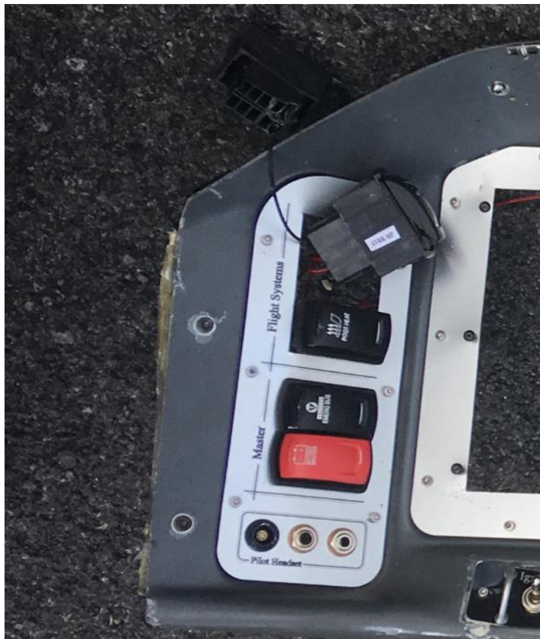
Photo 2 – View of master and essential bus switches (Photo courtesy of the pilot)
