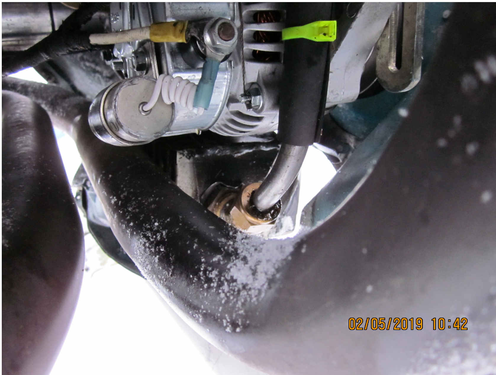
Photo 2 - Loose B-Nut Looking from the Side (FAA Photo)
