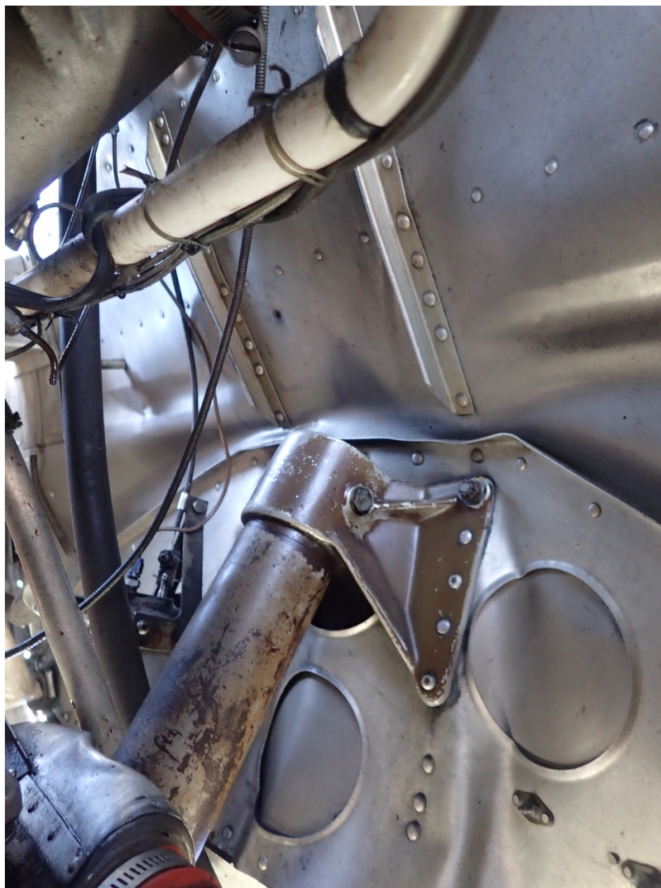
Photo 3 - N5020D buckled engine firewall.
