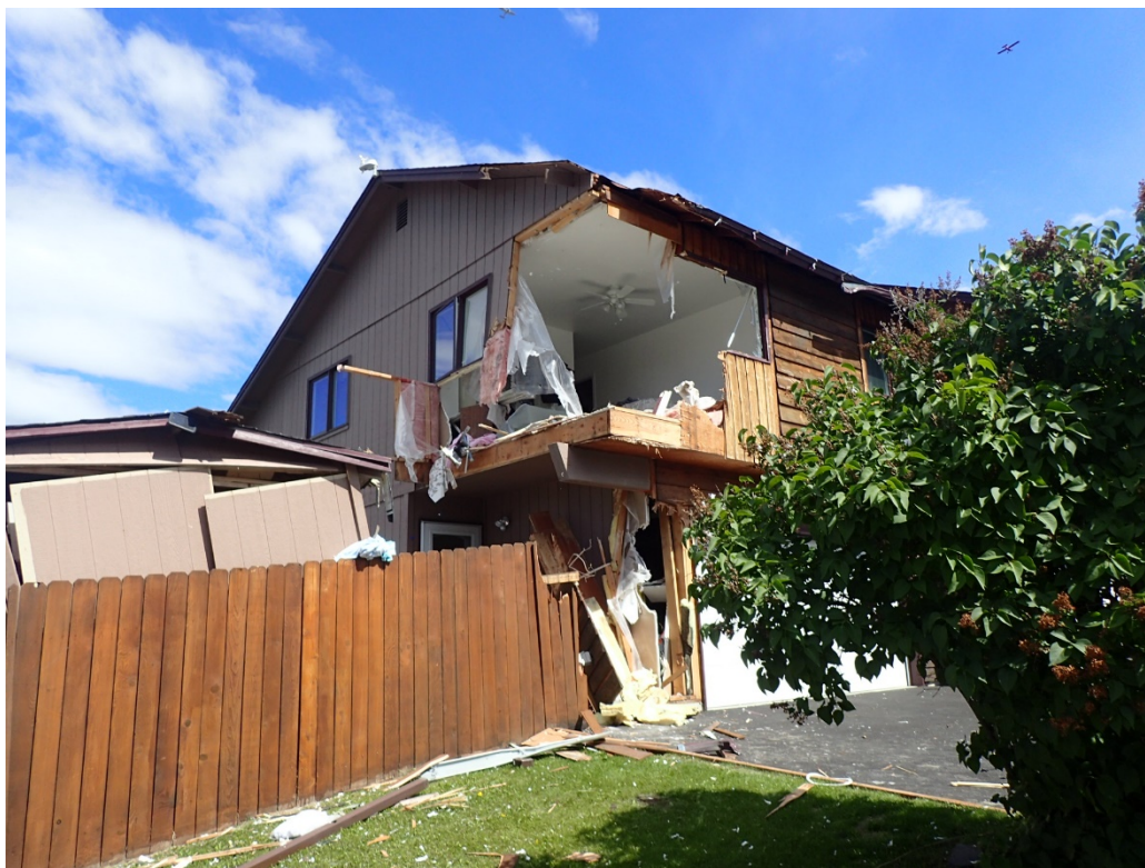
Figure 4. Damaged house and shed.
