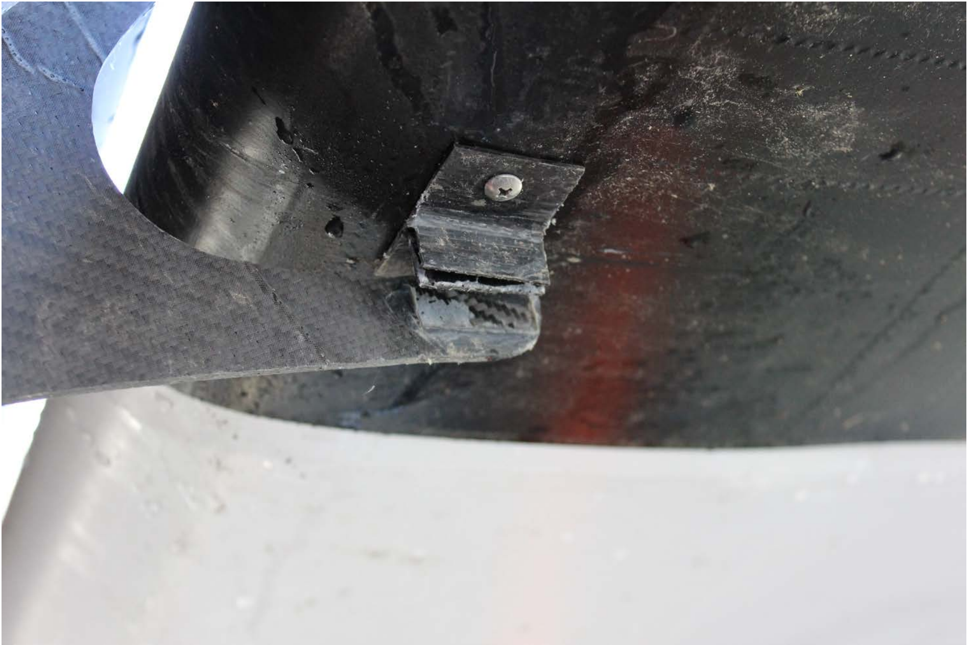
Photo 6 – Left wing leading-edge slat attachment bracket adhesive failure and a disbond at the attachment.
