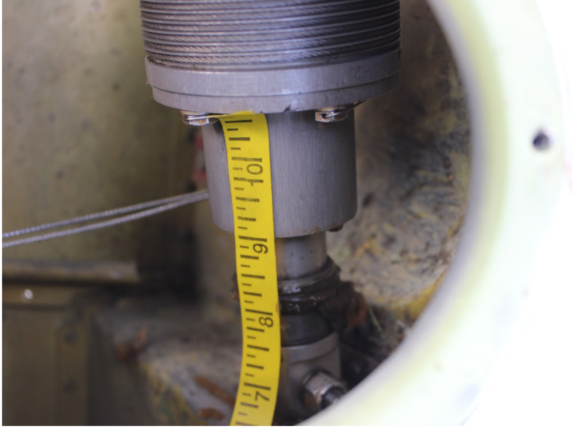
Figure 6: Measurement of the jackscrew
